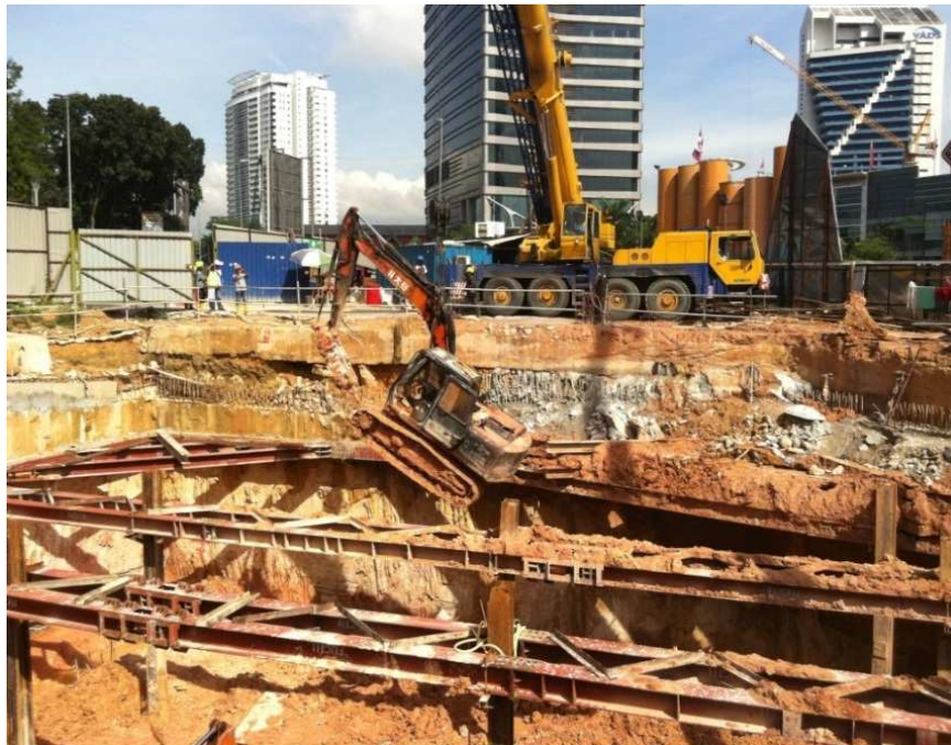
A small excavator had to be lifted out of the basement upon completion of the earthworks
